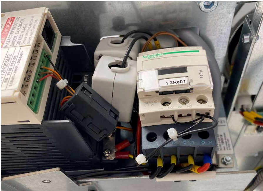
Column motor connections to 1.2RE01 (wire 1-3 and PE).
